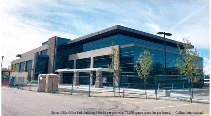
Harvest Hills Office Park Building B has 52 per cent of its 74,350 square space feet pre-leased. — Colliers International
